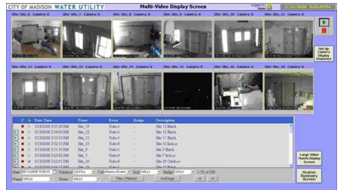
Figure 2: An operator at the water plant in Madison, WI, can quickly glance at video images from important areas of the process.
