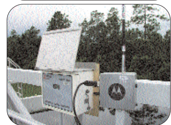
Mesh networking in a water treatment facility
