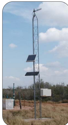
Real world example of a remote monitoring system using a slave/repeater design
