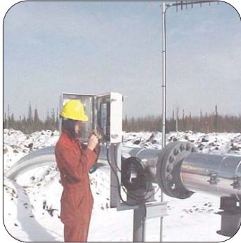
In remote and rugged conditions, reliability of your communications system is paramount
